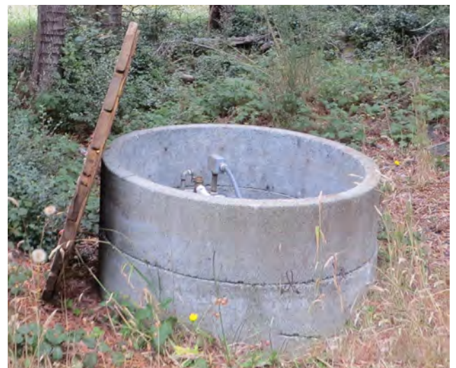
Well #2 Concrete Caisson Enclosure with Wood Lid
